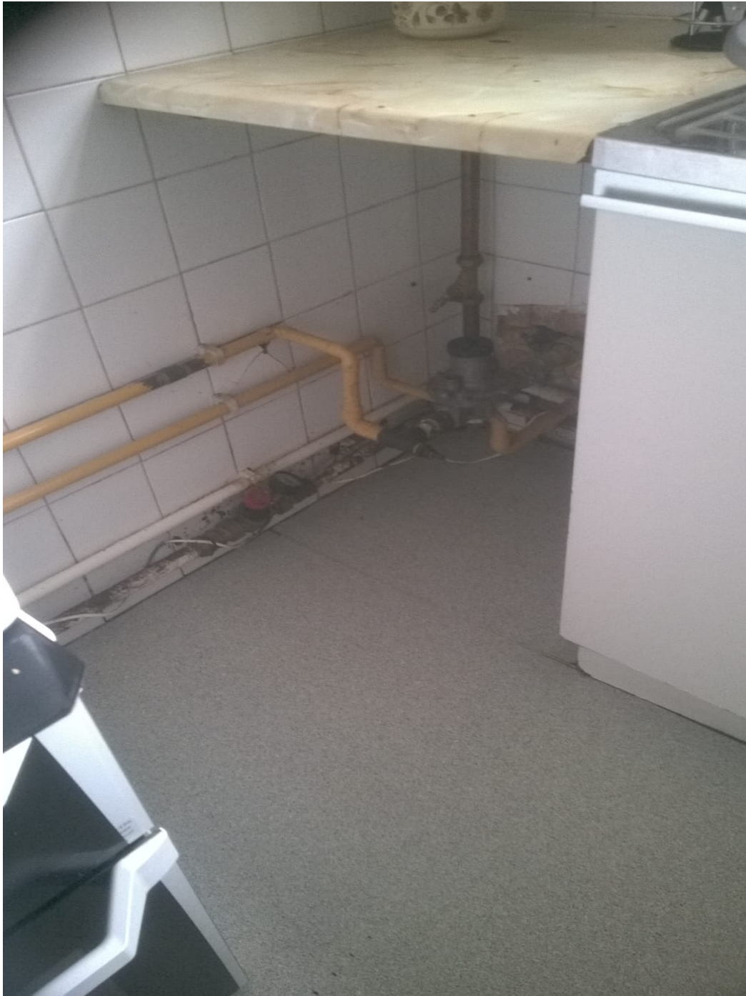
Kitchen (main building) This to be sectioned off after the works completed
